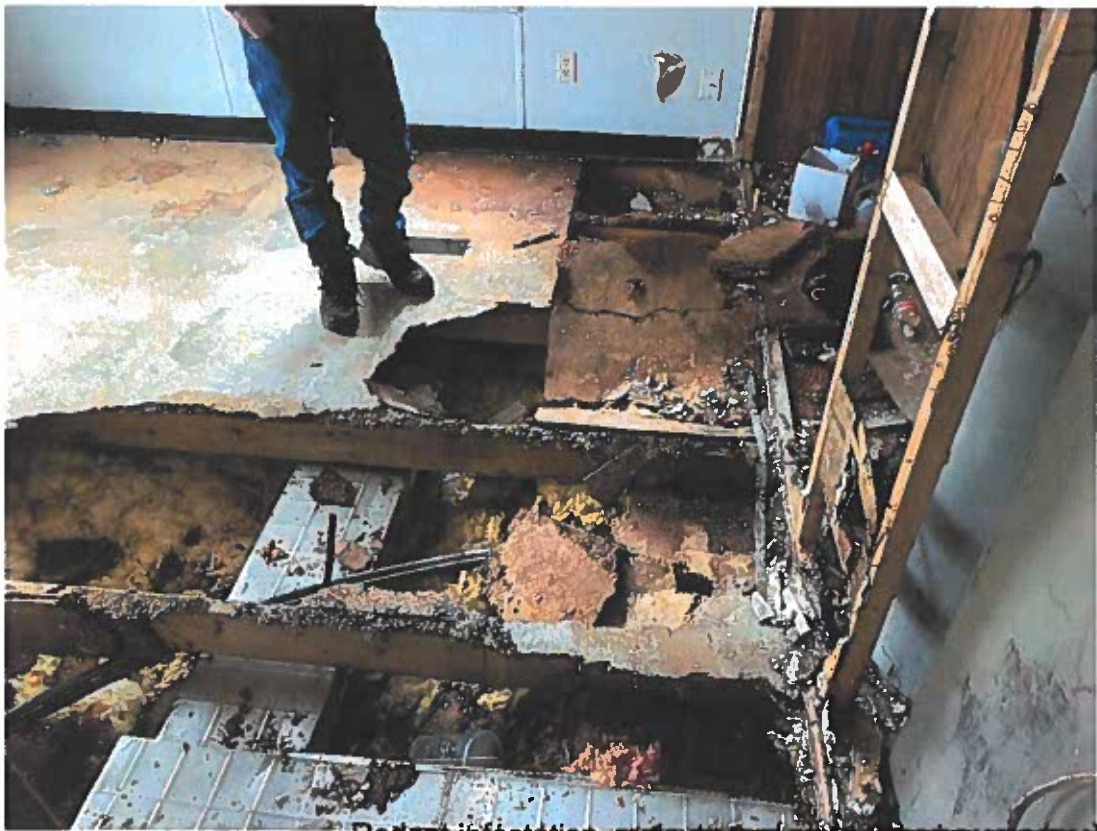
Rodent infestation, moisture and mold, missing smoke de
